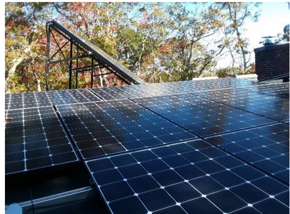
View of roof showing solar electric panels being installed and angled rack with solar hot water panels.
